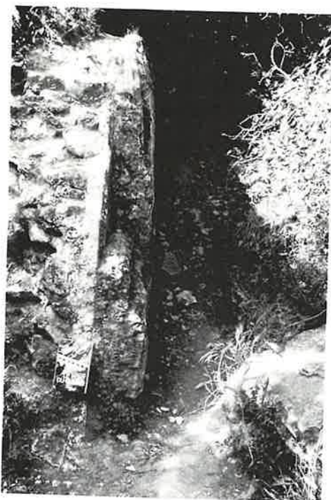
50. Nîmes: edge-on view of the sinter (calcium carbonate deposit) accumulated on sidewall (left) of aqueduct conduit, near the Pont du Gard. The sandwich-like layered structure of the accretion is clearly visible.
