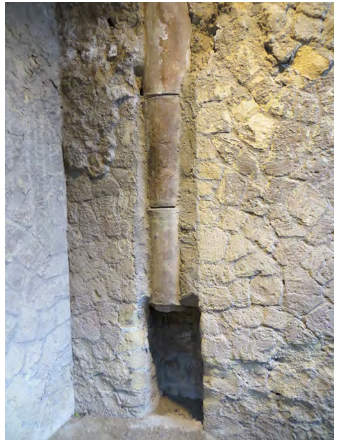
Figure 3. Herculaneum, House VI.29, leaky downspout.
